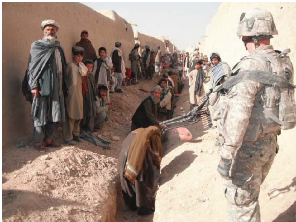
Local workers dig a sewage system in the village of Kandalay in Afghanistan.
