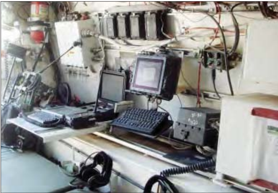
The workstation created for one Stryker is seen in its early stages. Various brackets and shelving had to be removed to free the system's eventual footprint.
