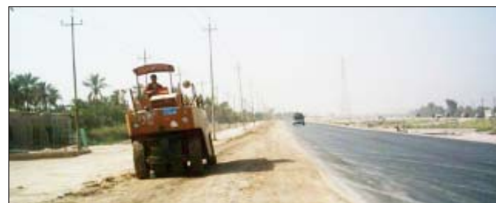
The Danish anti-IED project not only provided clearer lines of sight and a substantially decreased number of locations for IED emplacement, but also made it easier for local Iraqis to use the road for pedestrian and bicycle transport.
