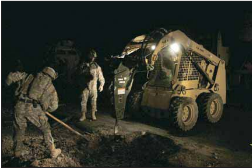
"Cleaning the roadsides was no easy task; we operated at night, during curfew, which allowed us to work unhindered from civilian traffic and during hours when attacks from insurgents were least likely. We literally began walking from the front gate of the forward operating base (FOB) down both sides of the road, loading pieces of concrete onto trailers and pushing trash far away from the roadside. We made good use of the armored combat earthmover (ACE) and Bobcat tractors."
